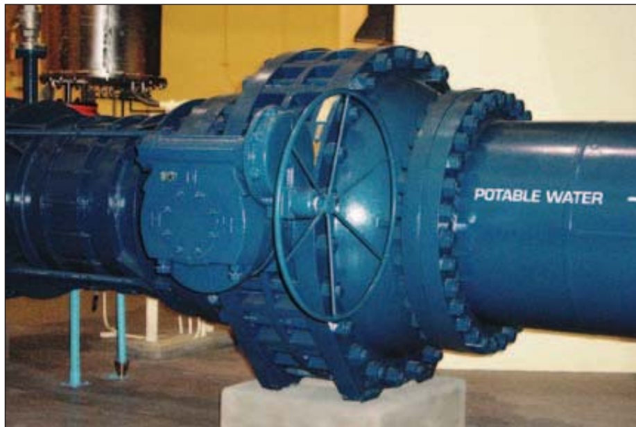
36" Rubber Seated Isolation Valve Application.
