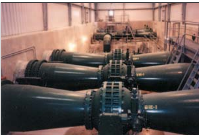
Ball valve in distribution pump station.
