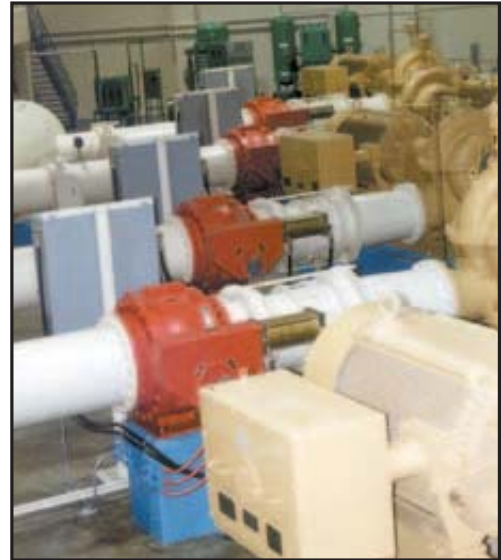
20" Metal Seated Ball Valves in Pump Control Service
